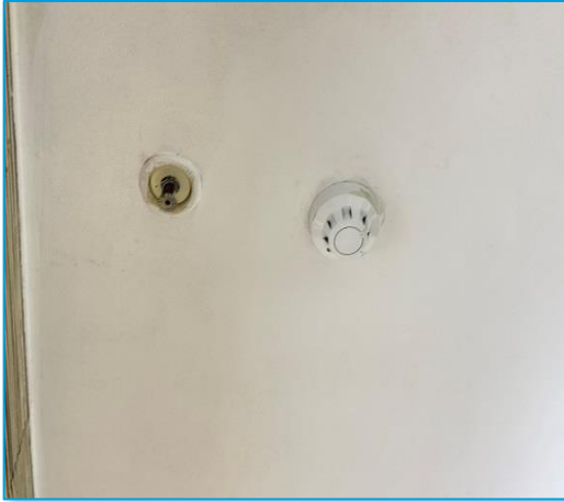
Sprinklers & Smoke Detectors
